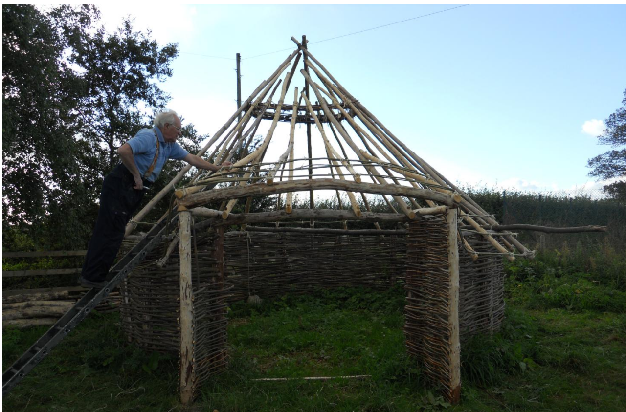
AND's reconstruction of an Iron Age round house in progress (Image Copyright: Brian Elsey)
